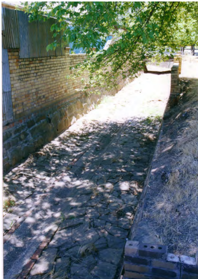
Photo 1.10: Significant brick and stone drain (former St Arnaud Creek), between Inkerman and Market Streets.
