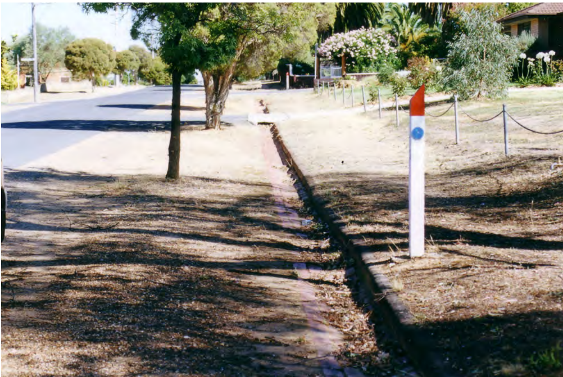
Photo 4.02: Queens Avenue (near Alma Street) Detail of early brick kerb and channel
