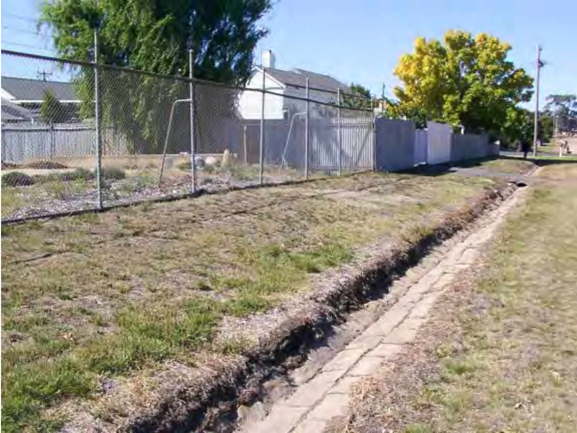
Photo 5.08: Detail of the early, open Stawell stone drain along the eastern end of Leslie Street, Stawell.
